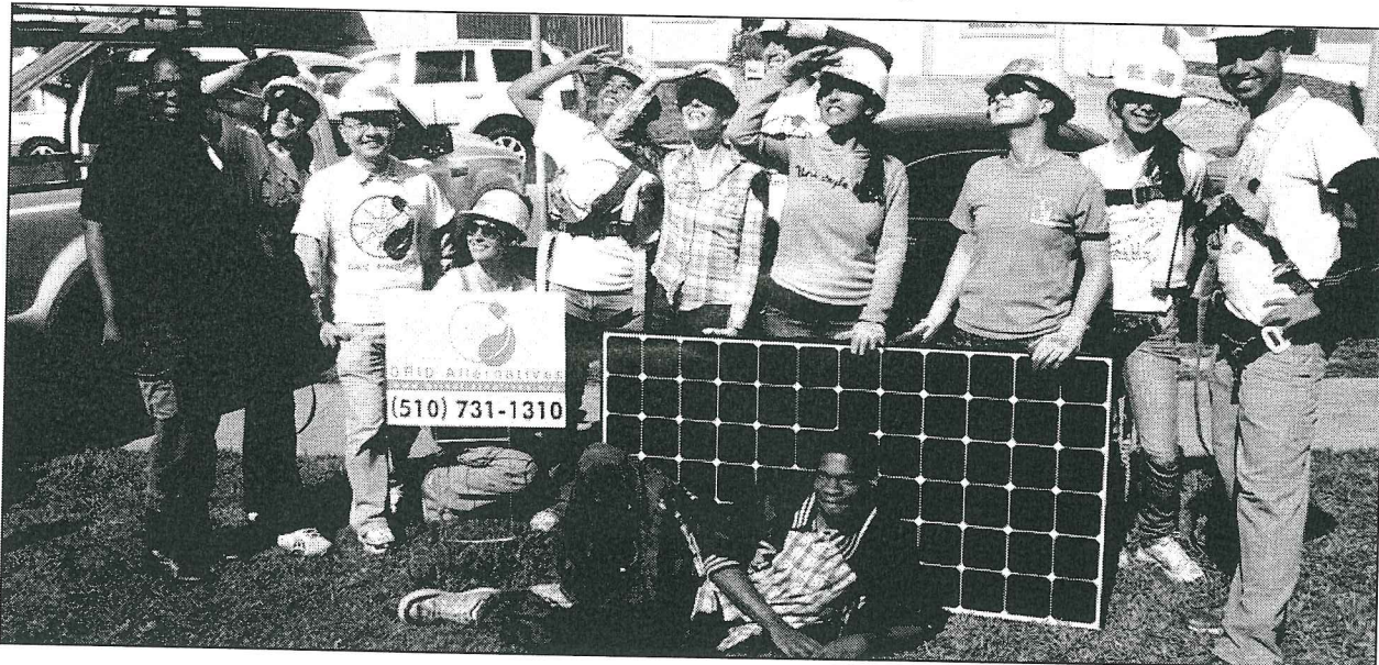
Volunteers from ERG installed solar panels for low-income families in Richmond, CA
